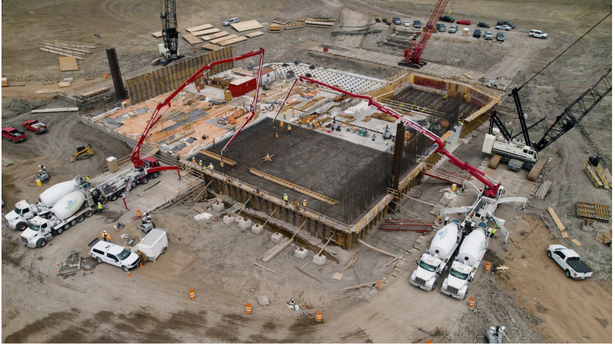
June 9, 2023: Red River Structure: Final of 4 mass concrete placements for 10-ft thick structure slab; also the largest concrete placement for the entire FMM Project. Photo from C Three Media
