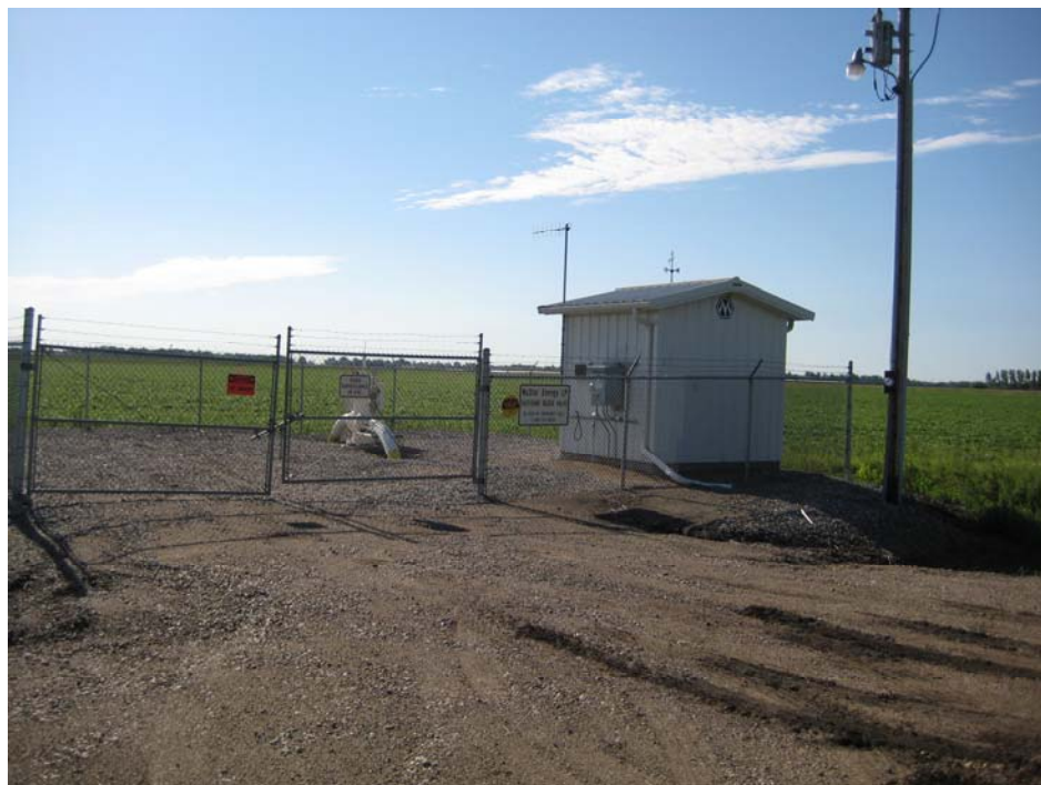
Figure 4 – Substation near intersection of 15 th Avenue and 21 st Street.
